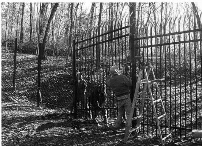
An eight-foot long section of the Shelta fence being racked into position
