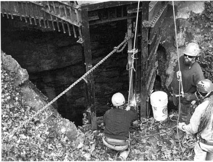
The inner door being cut off the west gate. From left to right are Tony Amundson, James DeForest and Scott Lynch.
